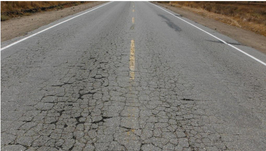
Lower Valley Road, Section 04, PCI = 12
